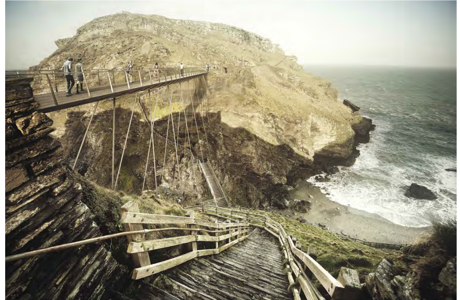
A STEEL GIRDER PRESTRESSED BY CABLES ANCHORED IN THE RAVINE. VIEW FROM THE EXISTING STAIRS ON THE LANDWARD SLOPE
